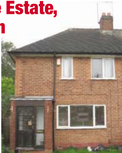
A HOUSE BEFORE REPAIR
